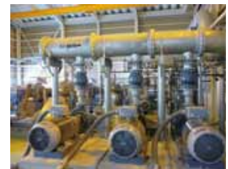
Lifting pump valves
