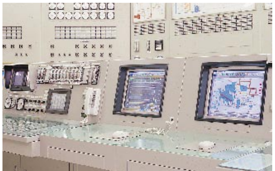
A Harmonas supervisory station installed in the central monitoring room at the Shinoro Waste Treatment Plant helps the city of Sapporo's staff keep tabs on plant operations.
