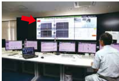
The monitoring screen of Advanced Critical Trend Monitoring for Safety is displayed on a large-scale monitor at the Water Purification Management Center so that the status can be checked at any time. If an abnormality occurs, an alarm is displayed on the monitor to alert the staff.
