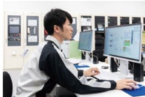
A savic-net G5 monitoring screen in the central monitoring room.
