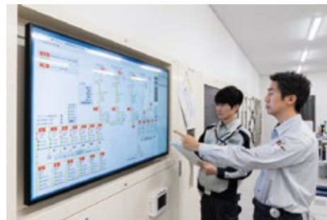
Checking the power outage contingency plan on a large savic-net G5 monitor that displays a summary diagram for incoming power.
