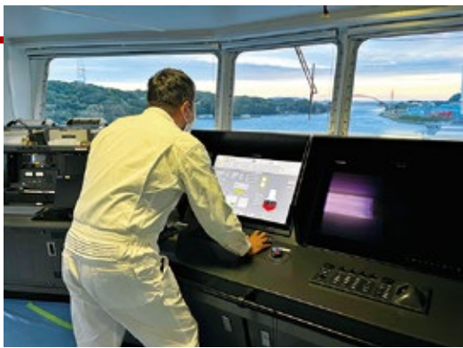
IAS (Harmonas-DEO) installed in the pilot house. The condition of the hard sail, which is automatically controlled based on wind conditions, can be checked in real time. In an emergency, the operator can also operate the system manually.
