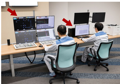
Monitoring screens for Azbil's DCS*5 system introduced as a DCS (left) and for the control valve maintenance support system (right).
