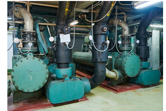
Chillers in the heat source machine room produce chilled water for air conditioning. The BEMS automates the start/stop of equipment according to schedules and controls the number of units that are operating.
