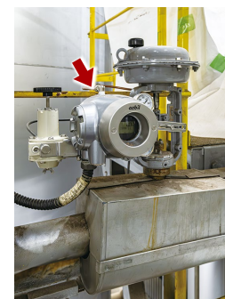
A smart valve positioner installed on another company’s control valve, which regulates temperature by injecting water into the steam used to turn power generation turbines
