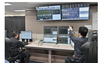
Harmonas-DEO monitors and controls the district heat supply plant. The system displays information other than the monitoring pane, such as weather data and security camera footage on the same screens, creating an environment where all operators can ascertain the overall situation at a glance.
