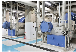
This electric turbo chiller produces chilled water, which is then supplied to customers through pipelines.
