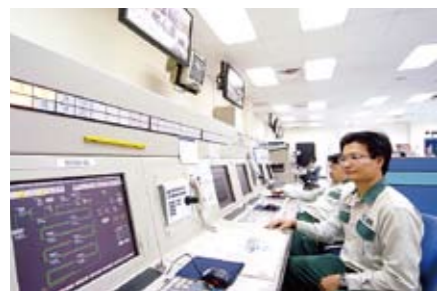
Harmonas-DEO installed in the central monitoring room monitors both Plant No. 1 and Plant No. 2.
