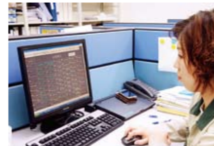
Client terminal of the TSS (Thin client Supervisory Server) server/client system installed in the office. MELS installed the TSS in order to check and operate the monitoring/control screen of the Harmonas-DEO from locations outside the central monitoring room.
