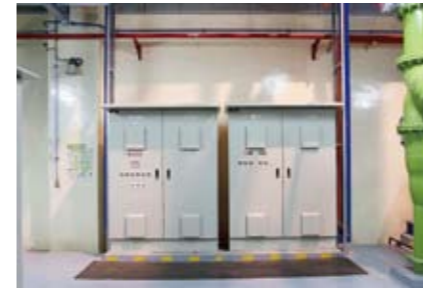
Control panels were newly installed in the plant. Cabinets store the controllers that control the chillers, pumps, and other equipment.
