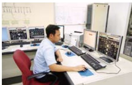
The Harmonas-DEO installed in the monitoring room enables centralized monitoring and control of chillers and other equipment in the plant.
