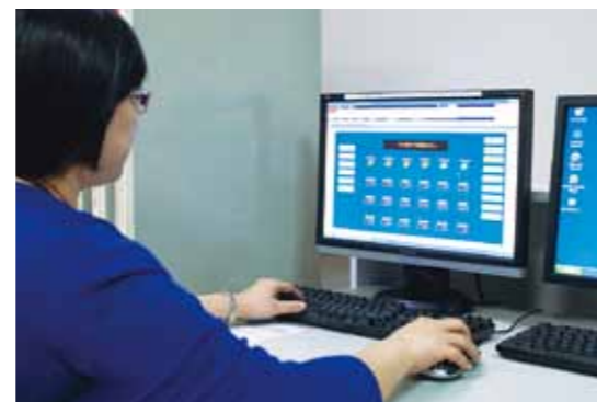
In the central monitoring room, the savic-net FX was installed as the BEMS.
