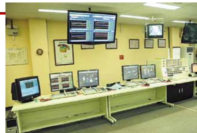
The Harmonas-DEO installed in the paraxylene plant.
