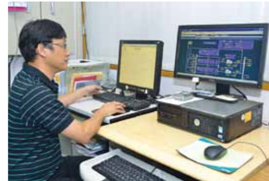
The monitoring terminals for the savic-net FX (right) and the EDS (left) in the monitoring room on the basement level of the library building. The operator can monitor and control the operation of the newly installed HVAC and check the energy consumption trend.
