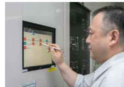
Azbil's Wall-Mounted BA System was selected for installation.
