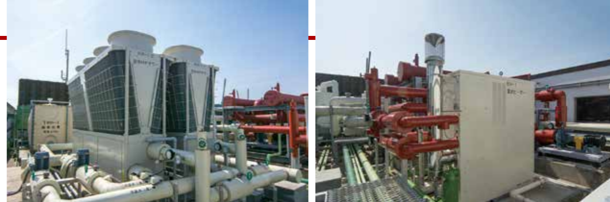
The air-cooled heat pump chillers (left) and hot water heater (right) installed on the roof of the Sakura City Museum of Art as part of the ESCO project are highly efficient.
