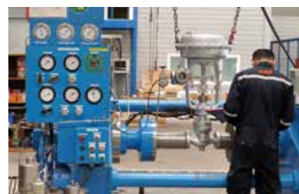
After the assembly, inspection, and repair of valves, a pressure-resistance test and airtight test are done to ensure quality.
