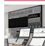
▶ Monitoring Monitoring and control systems
