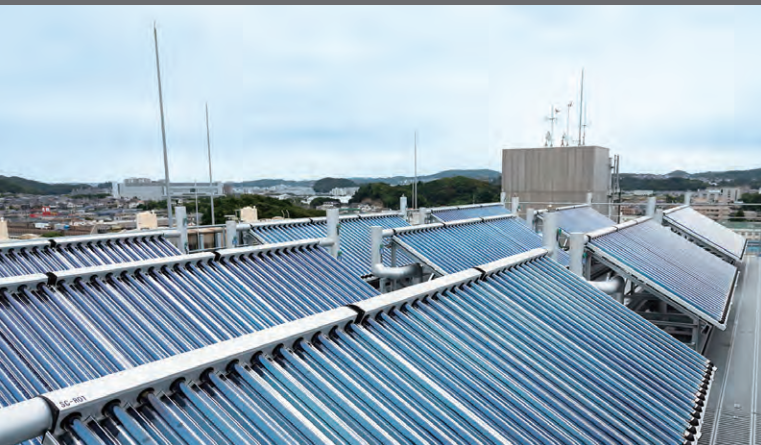
• The solar thermal energy system on the roof of Building 103
