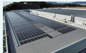
Solar power generation facilities at the Wakayama Factory
