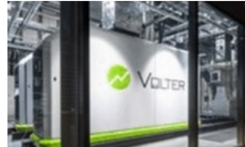
Volter: 40kW combined heat and power (CHP) unit fueled by woodchips
